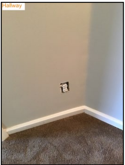
Outlet cover plates missing.
