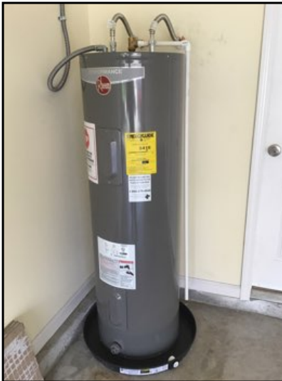
The water heater enclosure is functional.
