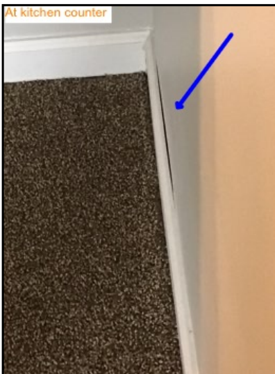
Loose Baseboards noted, recommend correction.
