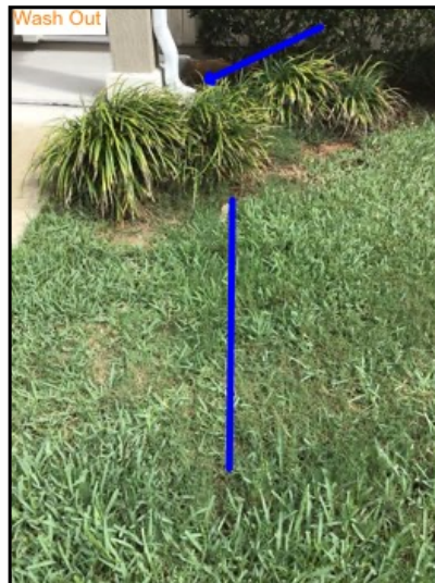
Tripping hazard noted due to gutter system runoff, recommend pipe installation to further prevent erosion.
