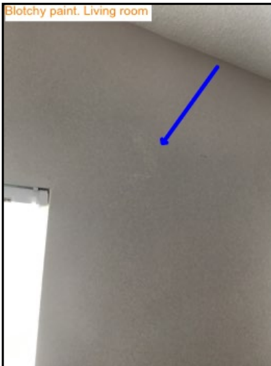
Blotchy Paint noted.
