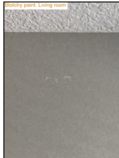
Blotchy Paint noted.
