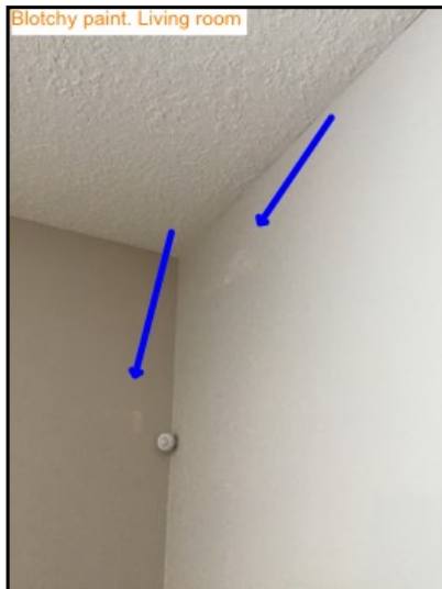
Blotchy Paint noted.
