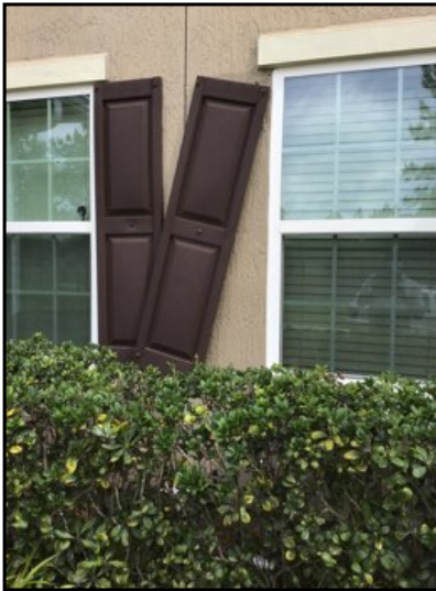
Loose shutters noted, recommend correction.
