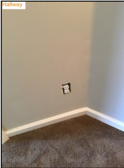
Outlet cover plates missing.
