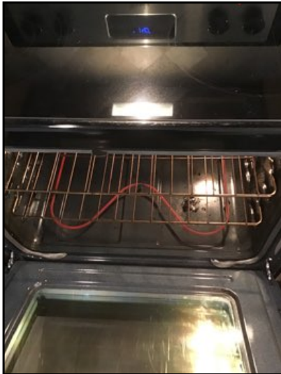
All heating elements operated when tested.
