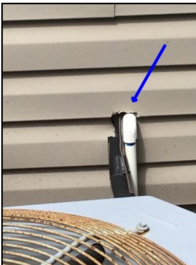
Recommend sealing gaps and voids as necessary.
