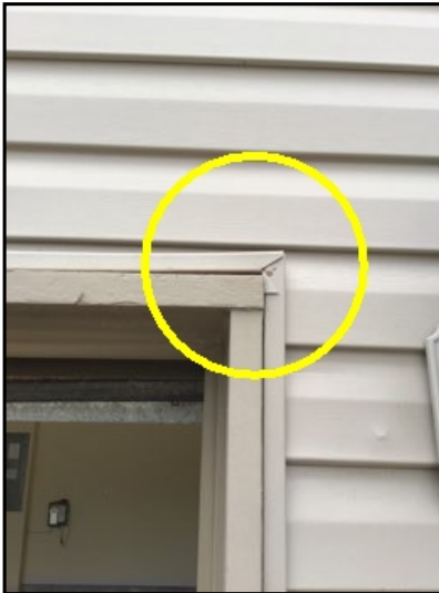
Loose trim Noted.
