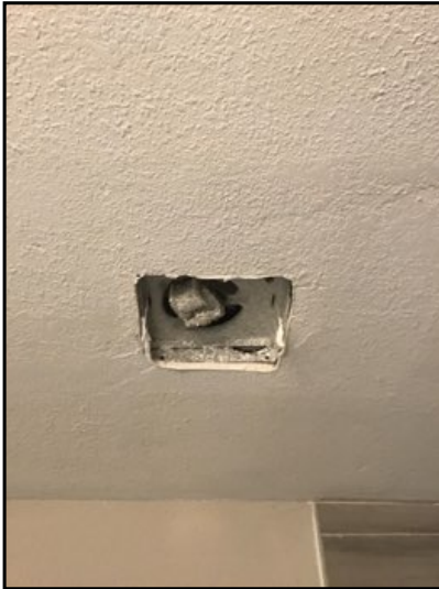
Installation is incomplete.
