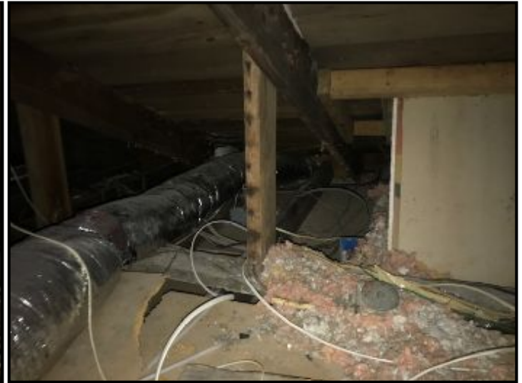
Insulation is sparse in some areas.
