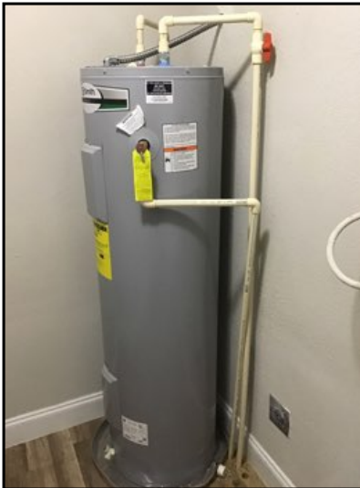
The water heater enclosure is functional.
