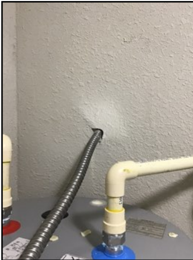
Recommend sealing gaps and opening to prevent air loss.
