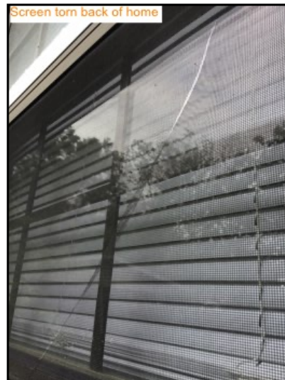
Some window screens missing and some damaged.
