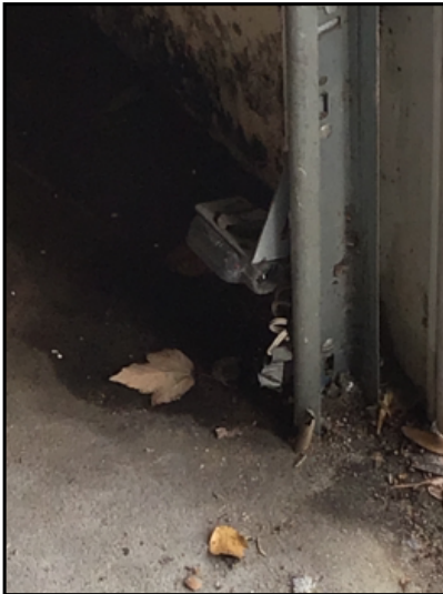
Inoperable due to Garage Door Opener malfunction.
