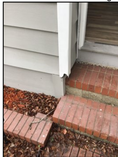
Vinyl siding damage. Recommend repair or replacement of damaged sections to keep moisture and insects from harming structure.
