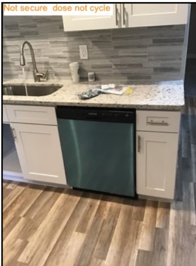
Unit is not properly fastened, recommend securing to countertop using the appropriate length screw to prevent tip from exiting top of counter causing damage.
