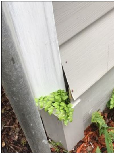
Loose/ damaged trim noted, suggest correction.
