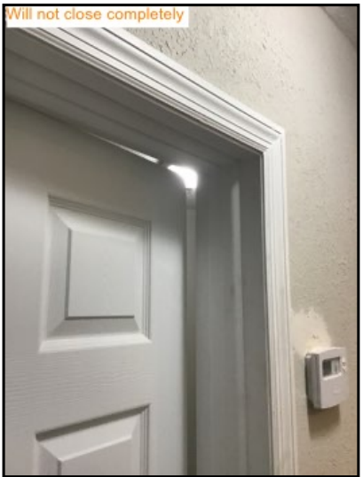
Doors not properly aligned, recommend correction.
