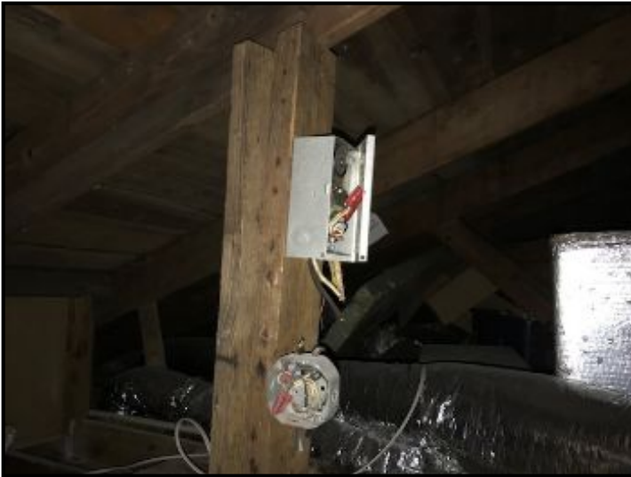
Electrical Box Covers missing or damaged, which is a potential shock or electrocution hazard.
