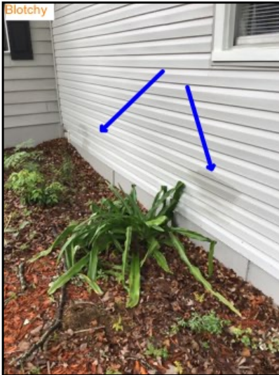
Blotchy painted noted.
