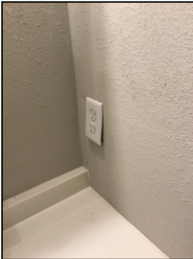
Outlet loose from the wall, recommend correction.
