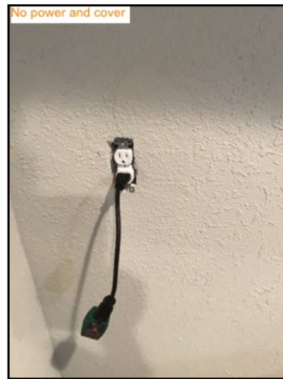
There was no power present.
