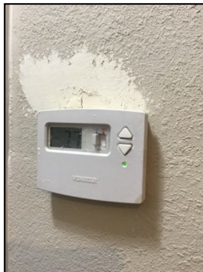
Thermostat does not appear to start unit, have furnace fully inspected by a licensed HVAC technician.
