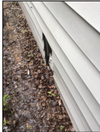
Vent screens noted as missing.
