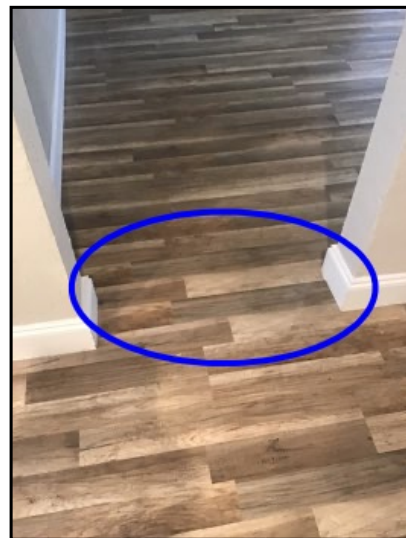
Some buckling noted.
