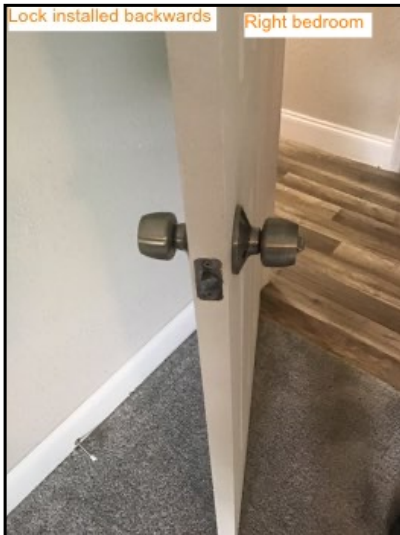
Lock(s) installed backwards, recommend correction for safety.
