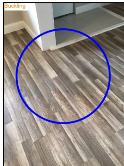
Some buckling noted.
