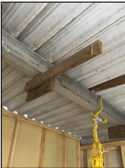
Recommend a qualified structural engineer review.
