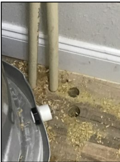
Minor damage noted.
