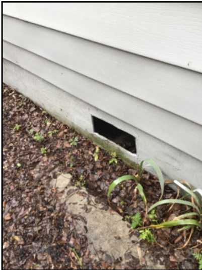
Vent screens noted as missing.
