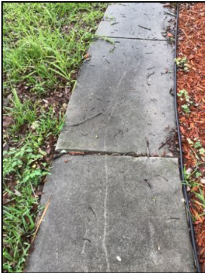
Moderate cracks in sidewalk. Repair and / or monitor for expansion and development of trip hazards.
