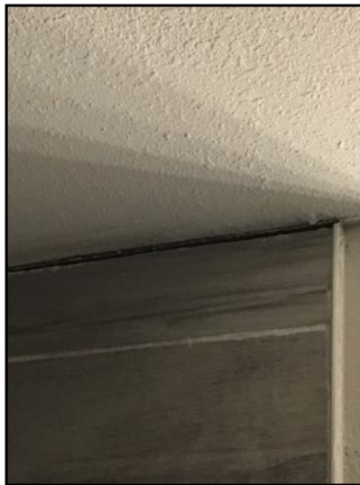
Recommend sealing holes & gaps to stop water infiltration into walls.
