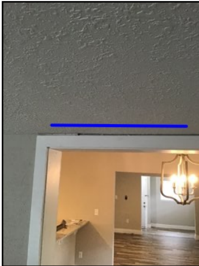
Recommend sealing gaps as necessary.
