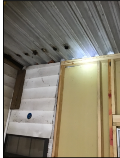
Garage drywall ceiling needs to be properly repaired.
