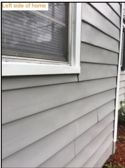
Loose/ damaged trim noted, suggest correction.
