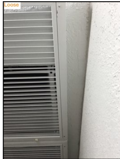
There is a loose return air grill noted.
