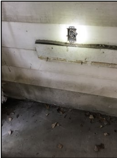
Outlet cover plates missing.
