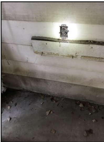
Outlet cover plates missing.
