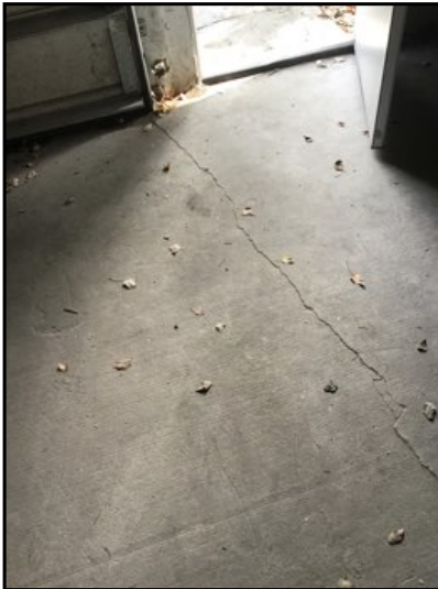
Common cracks noted.
