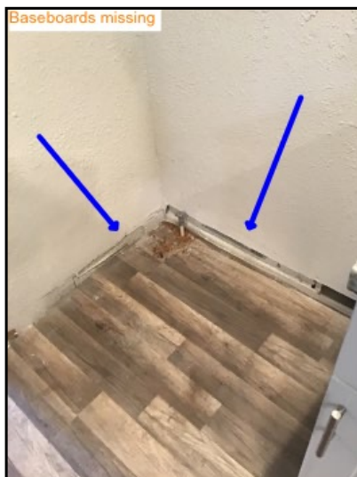
Incomplete installation noted, recommend finishing with baseboards or 1/4 round.
