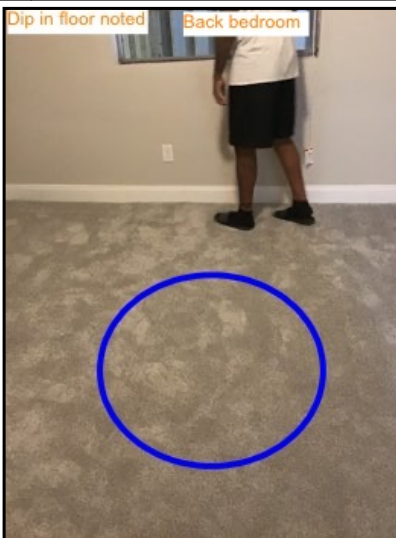
Low spot noted, recommend pulling carpet and finding the source!
