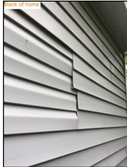
Vinyl siding damage. Recommend repair or replacement of damaged sections to keep moisture and insects from harming structure.
