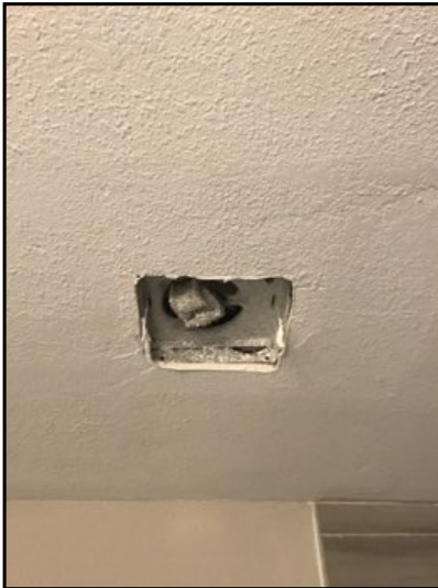
Installation is incomplete.
