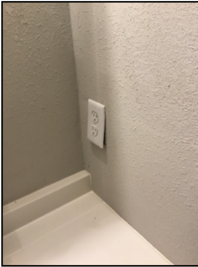
Outlet loose from the wall, recommend correction.
