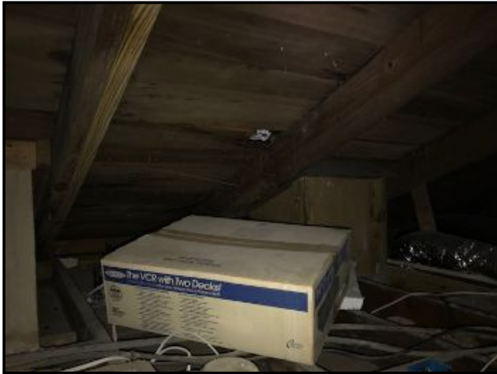
Insulation is sparse in some areas.
