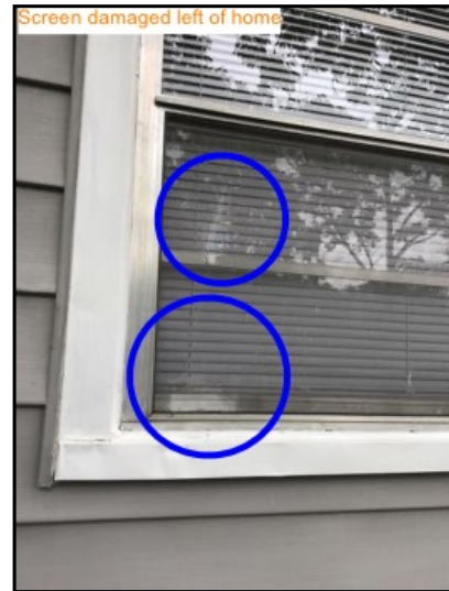
Some window screens missing and some damaged.
