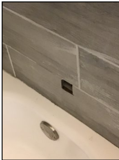
Installation is incomplete.
