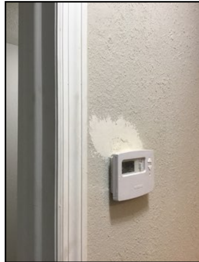
Past repairs made, not professional quality. May need sanding and repainting.
