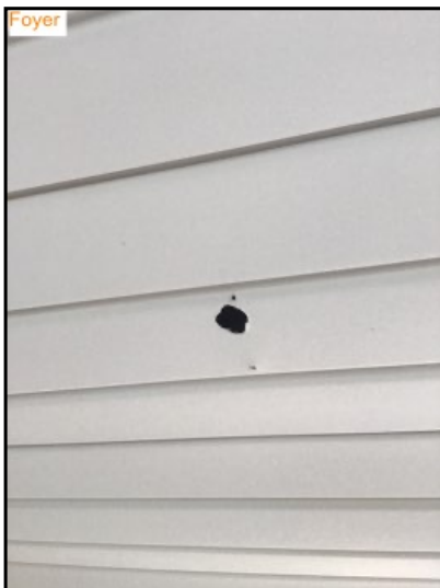
Recommend sealing holes and gaps to prevent air loss and insect entry.
