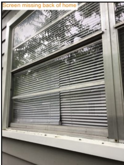
Some window screens missing and some damaged.
