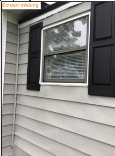
Some window screens missing and some damaged.
